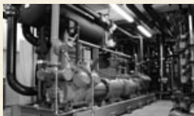
High efficiency heat pump system for a greenhouse for orchids
